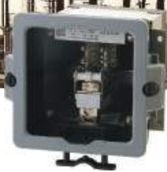
Auxiliary Relay in CSB Cabinet (92mm x 92mm)
