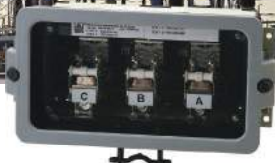
Auxiliary Relay in CSC Cabinet (186mm x 92mm)
